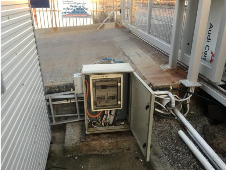
Electrical Shut-Off – Brighton Pier
